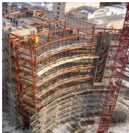
Mjärdevi Center under construction. Main framing and light steel for the exterior walls Photo courtesy of PPTH
