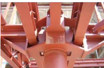
Bolted connection in a column placed in a corner between two cubes
